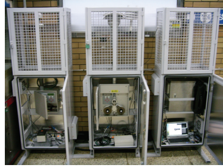
FIGURE 9: PM measuring instruments installed in “Jegi” subway station.
