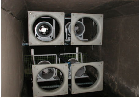
FIGURE 8: Ventilation fans installed at the natural ventilation point in the tunnel at “Jegi” subway station.
