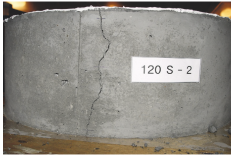
FIGURE 8: Cracking of ring specimen.
