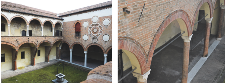
FIGURE 3: Inner yard of Casa Romei and zoom of the ground floor tie-rods.
