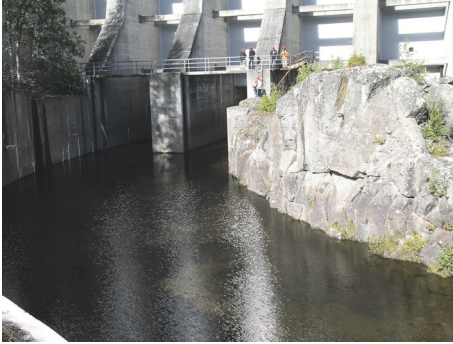
FIGURE 2: The bottom outlet seen from downstream, at a low tailwater stage.
