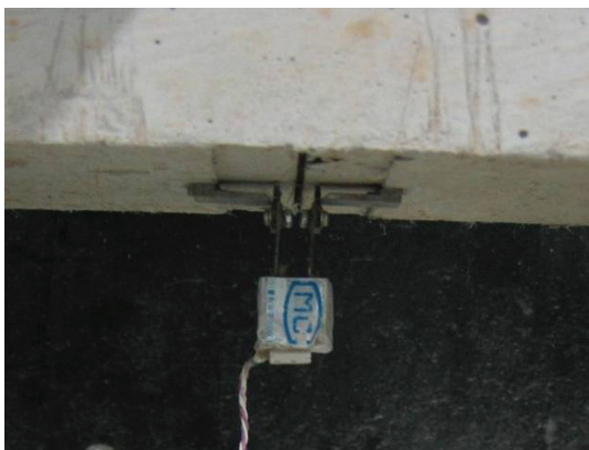
FIGURE 3: Crack opening displacement test.
