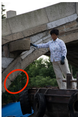
Figure 10. A ship passing the bridge with extreme carefulness and possibility of collision
