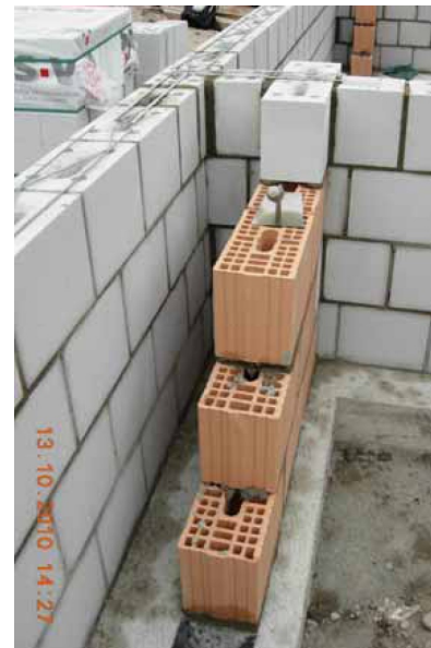
Fig. 3. Cross-section of the multilayer wall on the open-air test site Witaumatte (Thun, CH). The used materials are sand lime brick (left), brick (right) and insulating foam in between (not visible in this picture).
