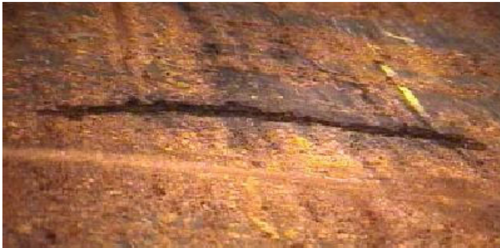
Figure 5: Example of Through-Wall Bleed-Out
