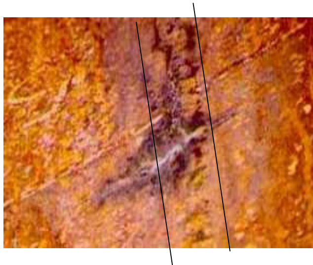
Figure 11: Visual Image of Crack in Upper Plate Vertical Weld, Riser 55
