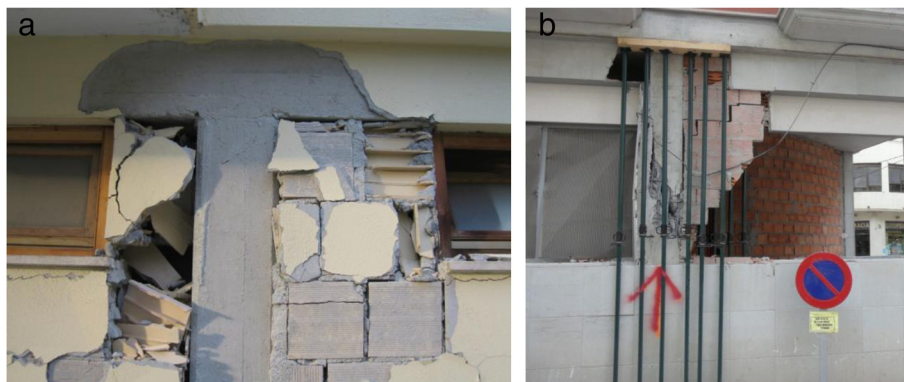
Figure 4 Column failure due to the presence of non-structural elements. Short column effect caused by window openings in residential building. (a) 2009 earthquake in L'Aquila, Italy and (b) 2011 earthquake in Lorca, Spain.
