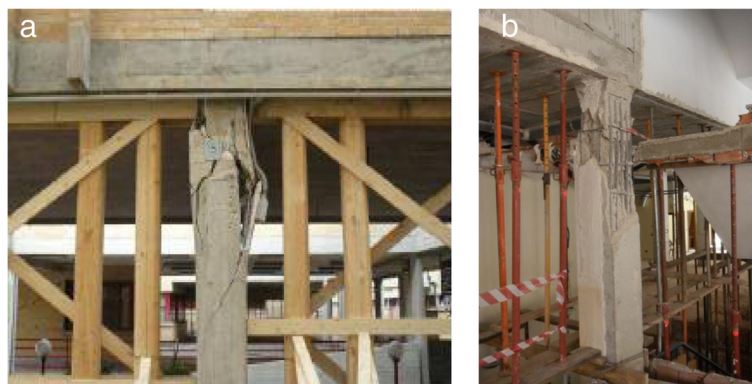
Figure 1 Flexural deficient behaviour in RC columns. (a) In the San Salvatore Hospital, in the 2009 earthquake in L'Aquila, Italy; (b) in a residential building, in the 2011 earthquake in Lorca, Spain.
