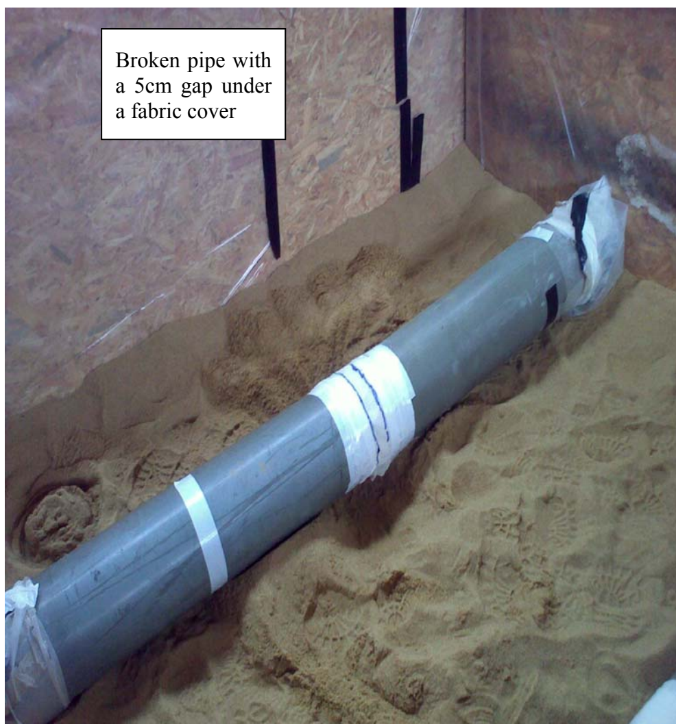
Figure 3.24: Broken pipe with a 5cm gap under a fabric cover
