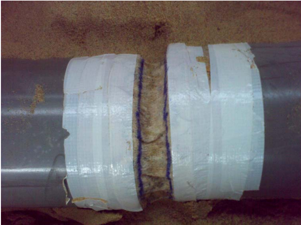
Figure 4.65: Test 6 - Broken pipe with a 5cm gap (sand prevented from passing through the gap by a fabric cover)
