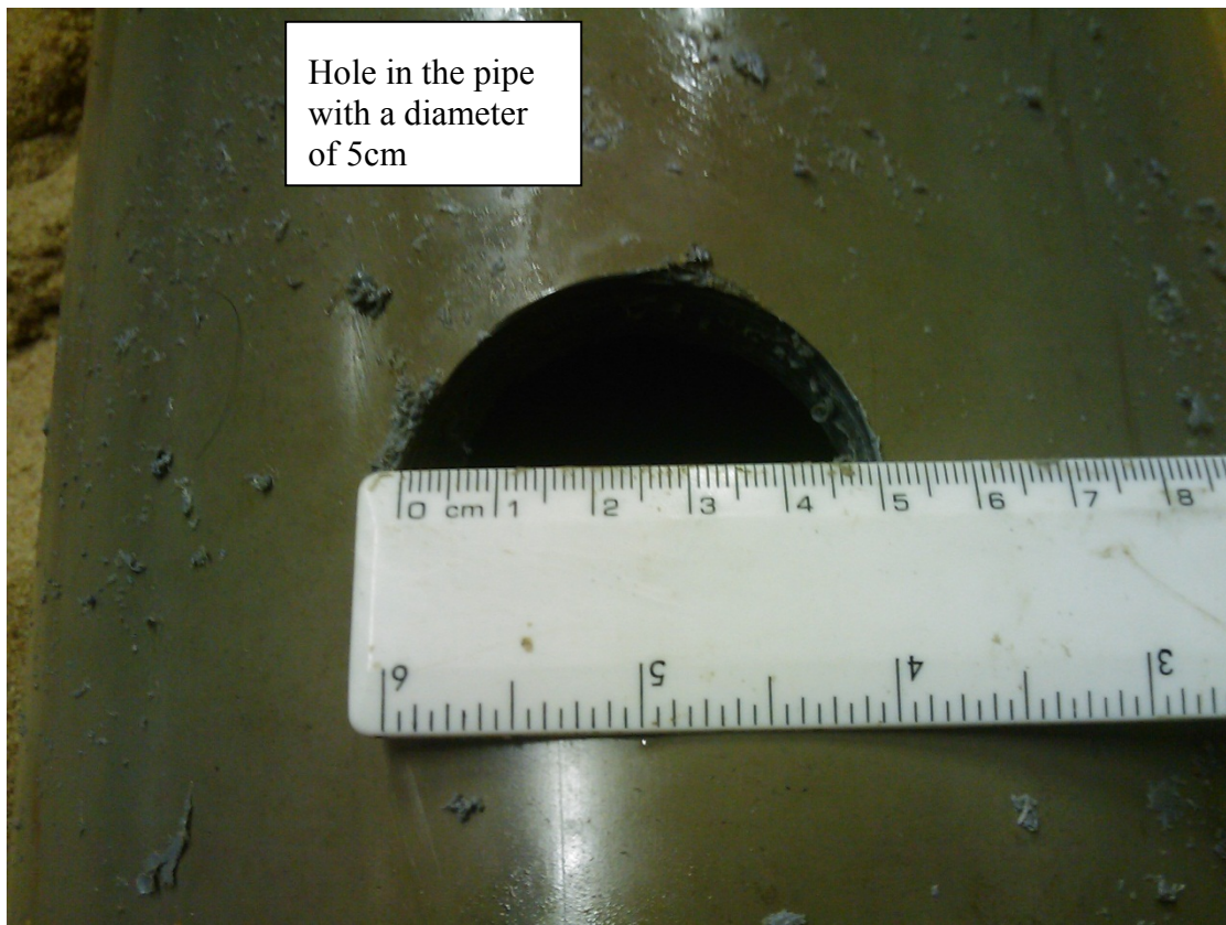
Figure 3.21: Hole in the pipe with a diameter of 5cm
