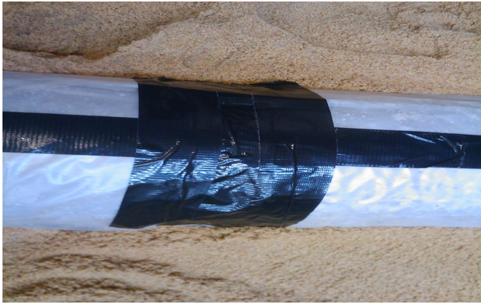
Figure 4.28. Test 2 - Broken pipe with a 5cm gap with a plastic cover
