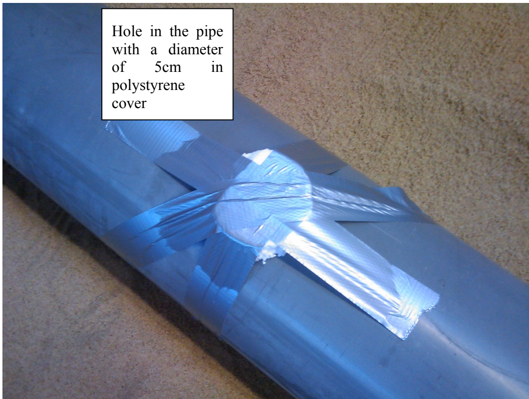
Figure 3.22: Hole in pipe with a diameter of 5cm gap in polystyrene cover
