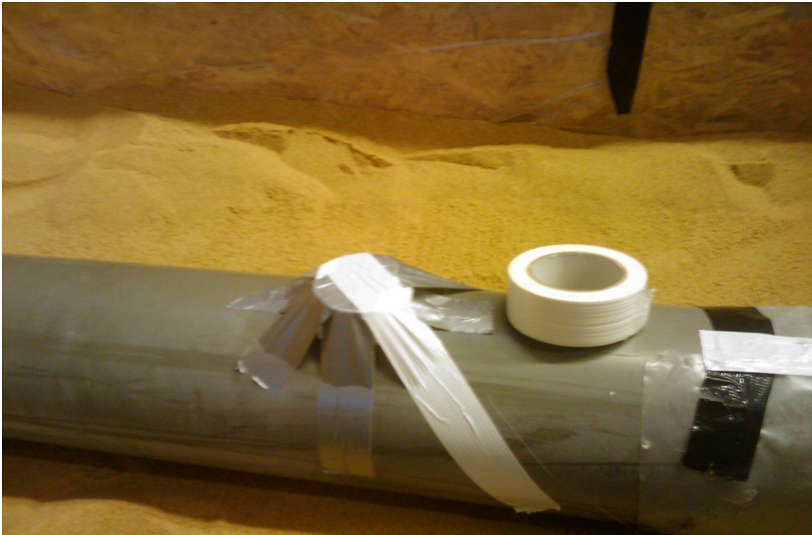
Figure 4.47: Test 4 – 5 cm hole in the pipe covered by polystyrene prior to being covered with sand
