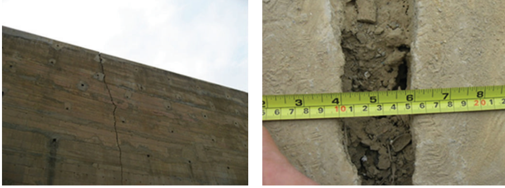
FIGURE 2: Cracks found on the retaining walls in Hanyuan.
