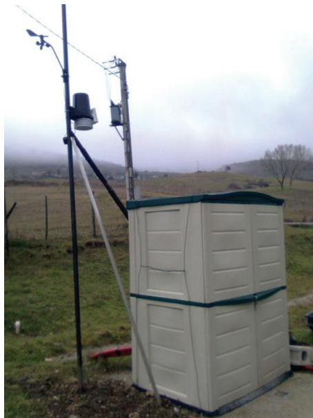
FIGURE 6: The weather station installed in the site.
