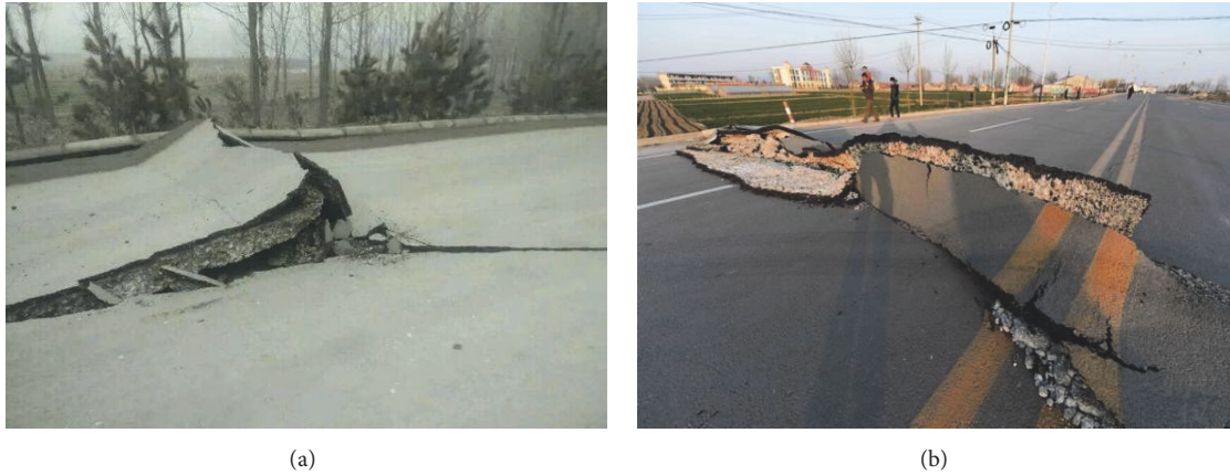
FIGURE 1: The damage of roads caused by the collapse of underground goafs in Shengda iron mine, where the vibration intensity was equal to an earthquake with the magnitude 3.1.
