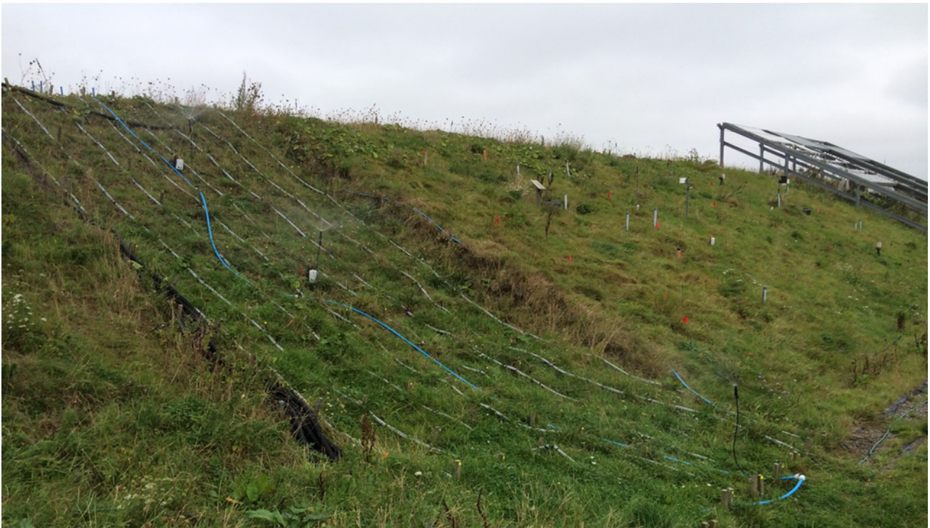
Fig. 1. BIONICS research embankment, Northumberland, UK. The facility has been used to understand earthworks behaviour in relation to climate and test new instrumentation approaches (photograph courtesy of R. Stirling, Newcastle University, UK).
