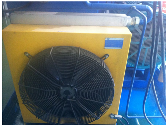
Fig. 4 The radiator in the cooling system
