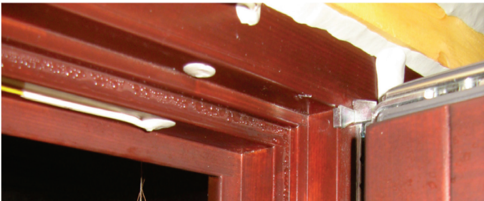
Fig. 3. Demonstration of condensation in gap between casement and window frame at exfiltration and 200 Pa pressure difference (upper part).
