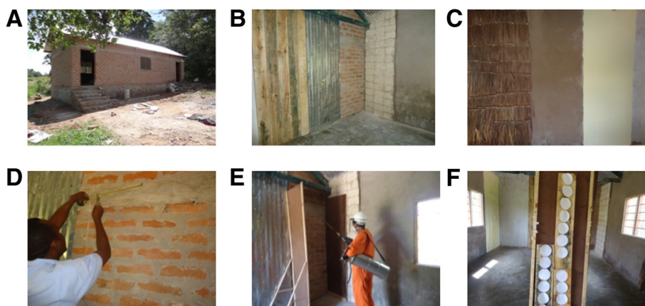
Figure 1 Design of the experimental hut and procedure used for spraying. A. An experimental hut with two rooms was constructed assembling nine different surfaces. B. Surfaces of wood, iron sheet, burnt bricks, limestone blocks and cement plastered walls are shown. C. Surfaces of palm thatch, mud daub and oil paint are shown. D. The substrates were fixed on the walls of the hut and demarcated to guide the spraying movement. E. Spraying on the tested surfaces was done using side edges to avoid overlap effect. F. Whatman paper was hinged on wood after being sprayed on tested surfaces.
