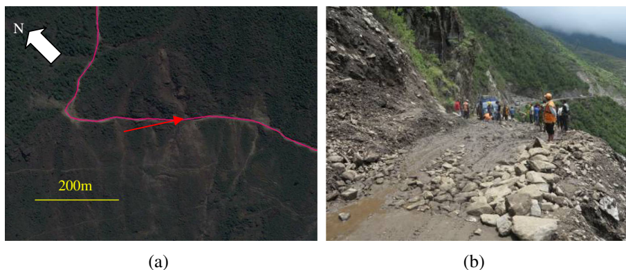
Fig. 5 A series of shallow, disrupted landslides blocking the Pasang Lhamu Highway. a Satellite image of 3 May 2015. b Field photo of 15 June 2015 (by Chong Xu, view to southeast) showing the road was blocked by a secondary landslide caused by a heavy rainfall. The red solid arrow in (a) shows the location of field photo in (b)
