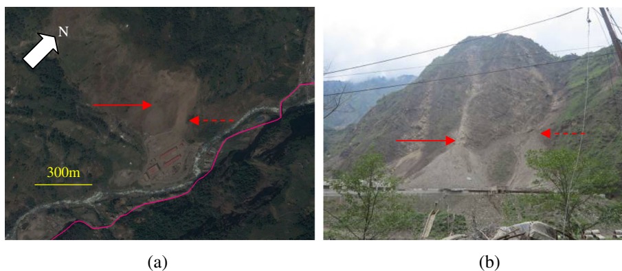
Fig. 4 Rockfalls on the upper slope of an inspection station of Nepal. a Satellite image of 4 May 2015. b Field photo of 14 June 2015 (by Chong Xu, view to northwest). The solid and dotted arrows in (a) and (b) indicate the same places, respectively
