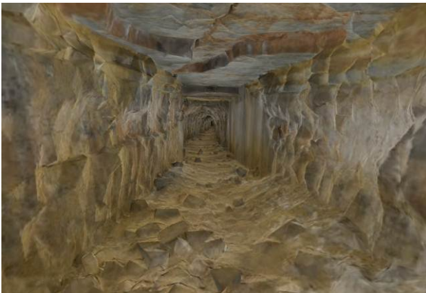
Figure 9. The final photorealistic 3D model of the tunnel, with the texture applied over the sharp optimized 10 cm mesh.
