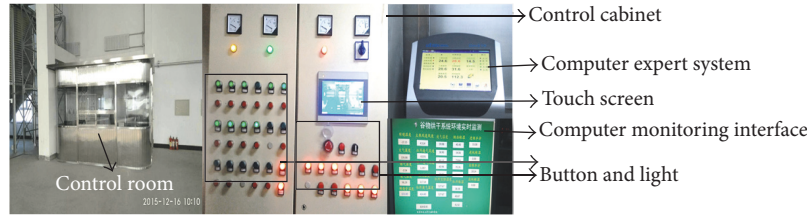
FIGURE 3: Controlling situation and equipment for the IRC grain dryer.
