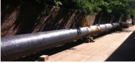
FIGURE 6: The pipeline for pull-through test.
