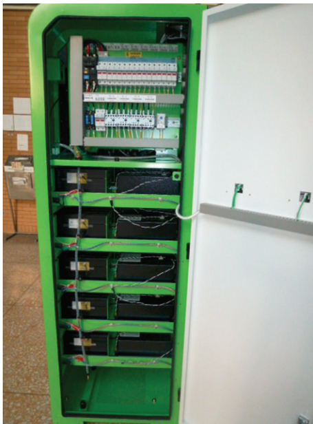
FIGURE 20: Completed RFID sensing system for BES.
