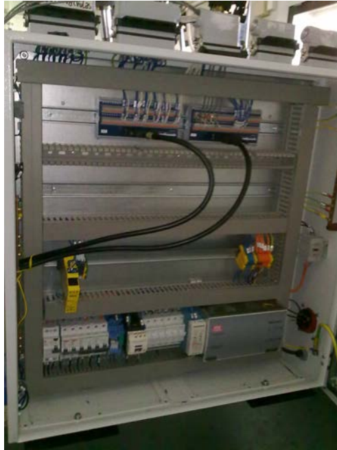
Figure 3.26: Electrical cabinet after reorganization.
