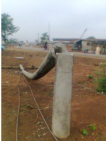
Plate 1: Fracture at 1,200 mm
