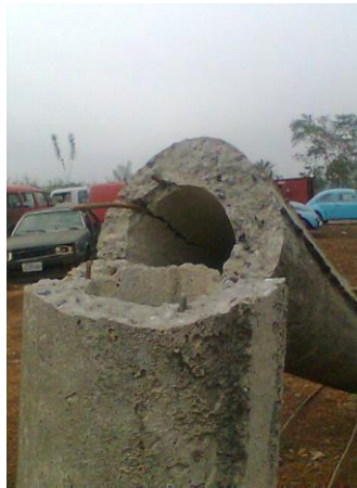
Plate 2 Clean fracture at 900mm
