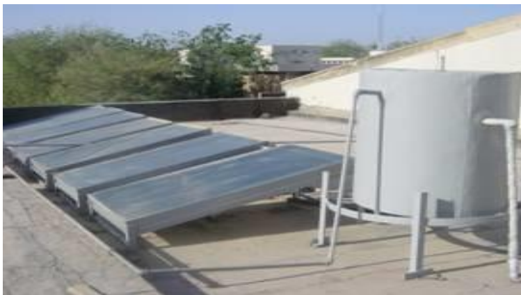
Figure 2.11. Community based solar water heater by SERC in Sokoto state
