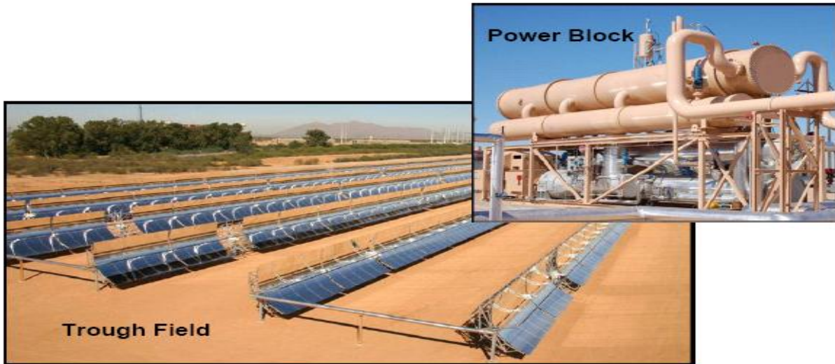
Figure 2.7: Trough field located at Saguaro Power station in USA
