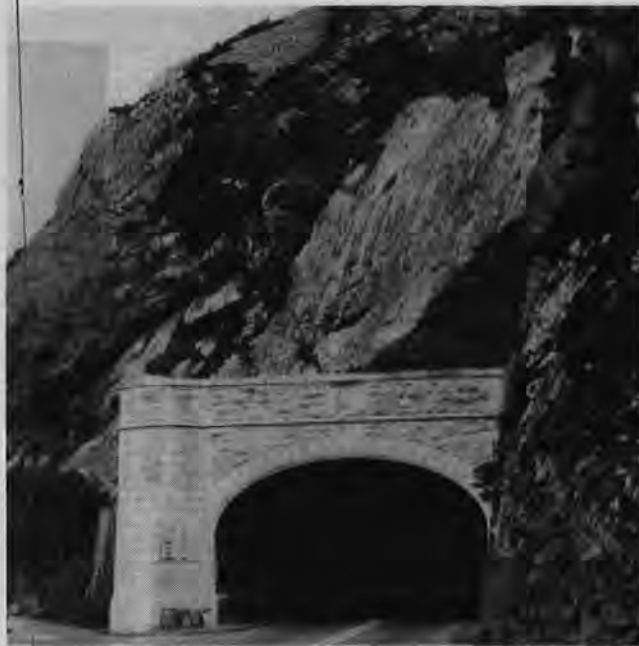
Fig. 8 Tunnel portal with rock slope failure
