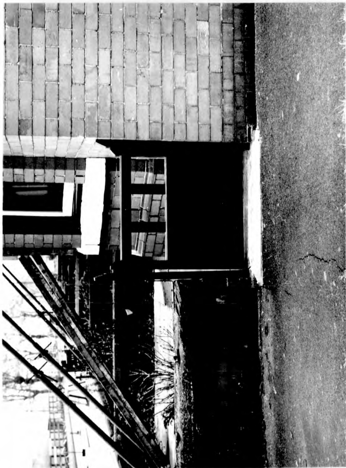
PLATE 6.2 STRUCTURAL DAMAGE AT SECTION B
