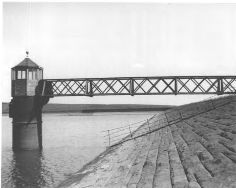
Photograph.5. Tower on 12.6.57. Top water level is just below the flange on the base of the tower. Distance from flange to water level shown is about 5 ft. (1.5 m.).
