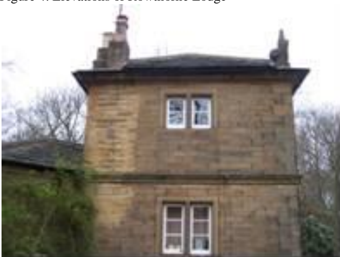
Figure 5: Stone decay along route of flue
