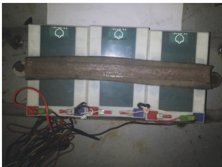
FIGURE 6: Sealed lead-acid batteries connected in series.
