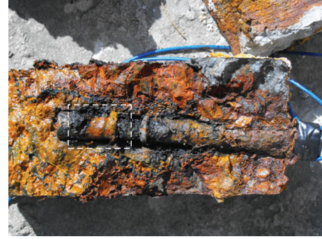
FIGURE 9: Corroded bar from FBG sample.
