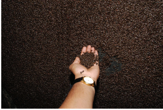
FIGURE 1: Aggregated beetles on the wall of a residential building.
