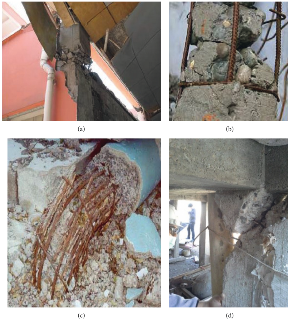
FIGURE 2: (a) Poor reinforcement detailing in Sichuan [20]. (b) Poor quality concrete in Sichuan [21]. (c) Collapsed column with inadequate lap splice length and widely spaced transverse bars in Gujarat, India [22]. (d) Poor reinforcement detailing in Chiang Rai [23].
