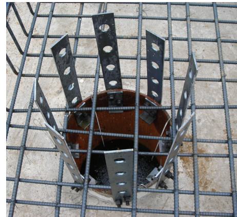
(c) Construction example of the proposed perfbond shear connector for steel pile cap strengthening
