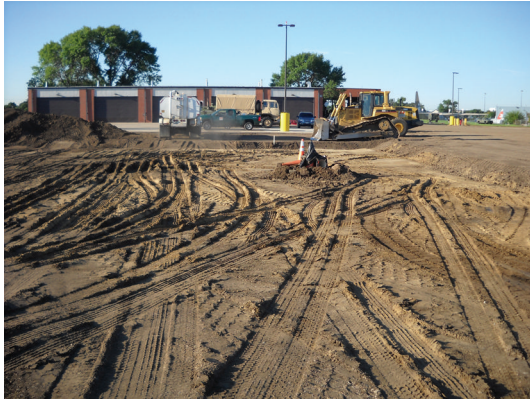
FIGURE 3: Photo showing typical rutting observed following proof rolling of the existing subgrade.
