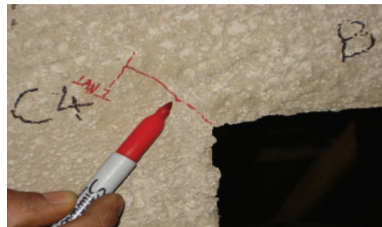
FIGURE 10: Shear crack in the column of the SDA concrete frame after test sequence 1.
