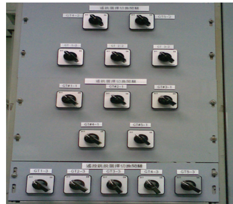
FIGURE 7: Generators tripping control panel of the first-stage SIPS.
