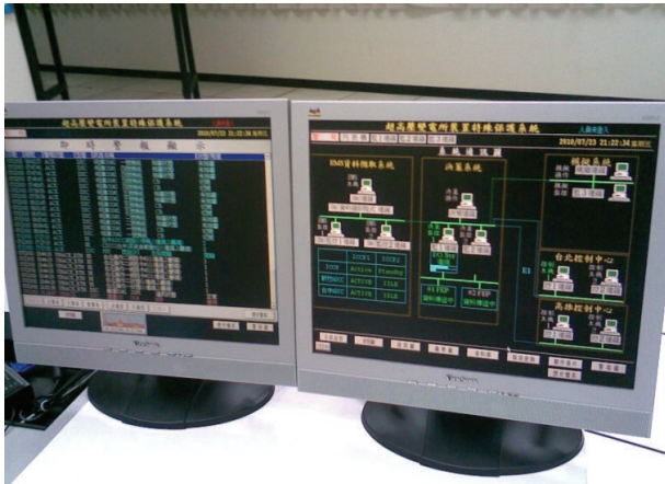
FIGURE 11: The second-stage SPS consoles sited at Taipei CDCC.
