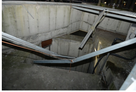
FIGURE 1: An accident that occurred in 2014 involving the collapse of ventilation covering [2].
