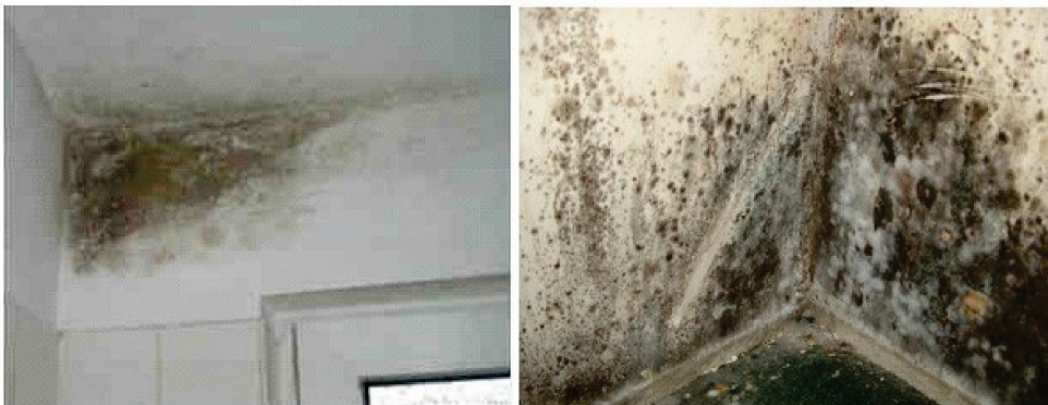
Fig. 2. Dampness, fungus and black mold on walls and ceilings.
