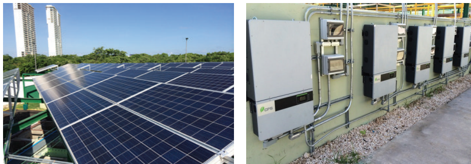
FIGURE 13: PV facilities of JAPAY in Merida city.
