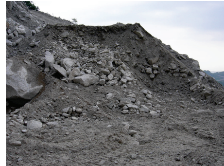
FIGURE 4: Granite quarry waste detail. The different, casual grain size distribution compromise the stability of the coarse volume.
