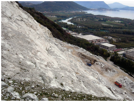
FIGURE 9: The uncovering of granite substrate thanks to mechanical equipments. The material is transported to the plant, located just below the slope (on the other side of the street).
