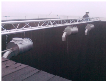
Fig. 2. Top of a quench tower with Mohrhauer's probes installed.
