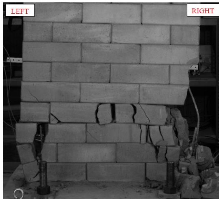
Figure 2: Wall 4 flexural failure characterized by spalling at the wall toe due to buckling of the vertical rebar (Stirling 2011)
