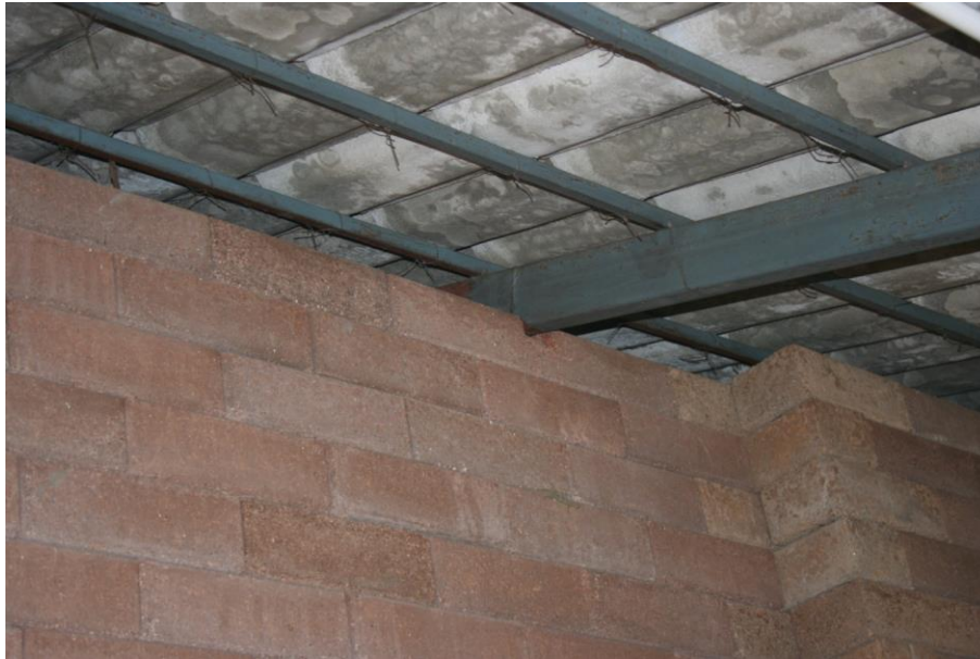
Figure 17: Rafter keyed into wall with no mechanical connection
