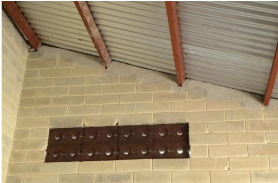
Figure 18: Rafter embedded in concrete layer with sideways blocks used for ventilation (Photo credit Co-op Ville Rehabilitation Project)
