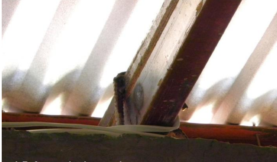
Figure 19: Protruding bar hooked over rafter (Photo credit Co-op Ville Rehabilitation Project)
