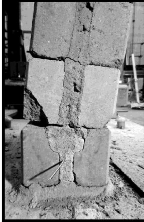
Figure 3: Out of plane rotation of an unplastered wall due to gaps in blocks (Herskedal 2012)
