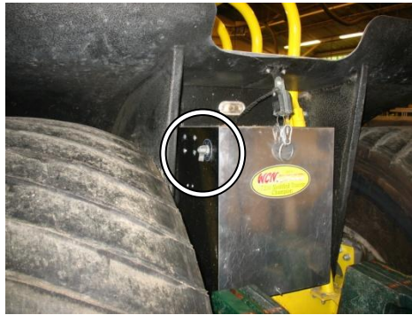
Figure 34. Main power switch.
