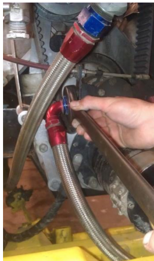
Figure 44. Fuel supply line.
