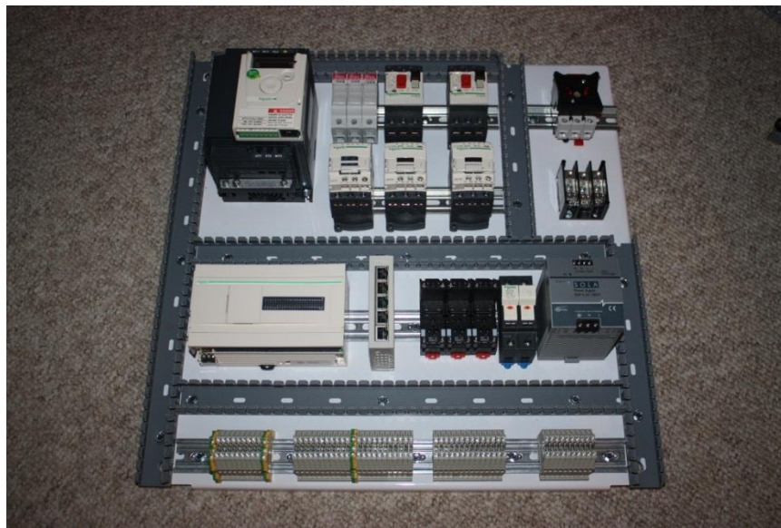
Figure 15. Subpanel with all electrical components mounted.
