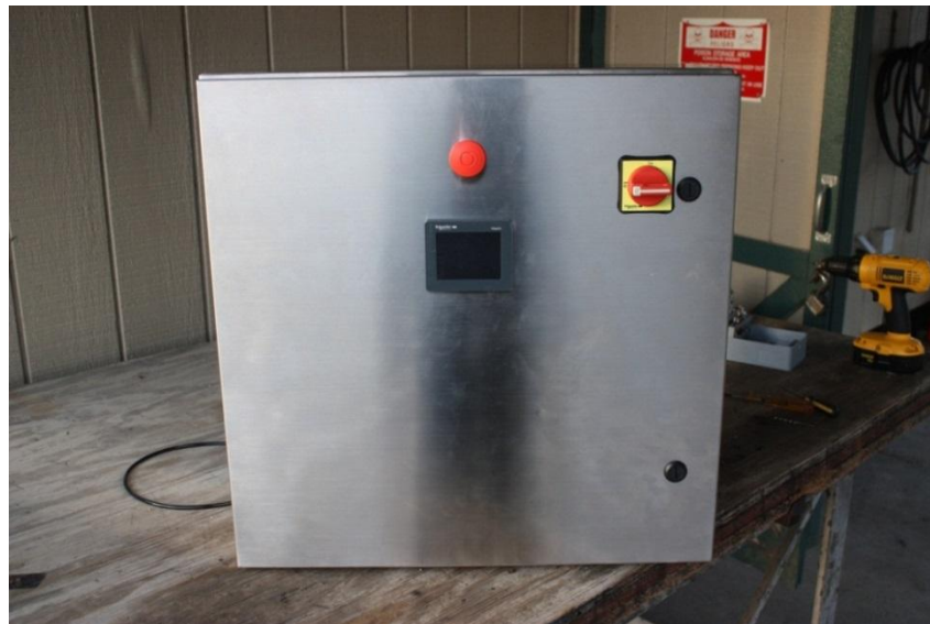
Figure 17. Panel with touchscreen, emergency stop button, and disconnect switch mounted.
