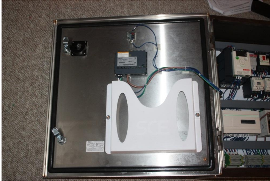
Figure 18. Panel with touchscreen and emergency stop wired up.
