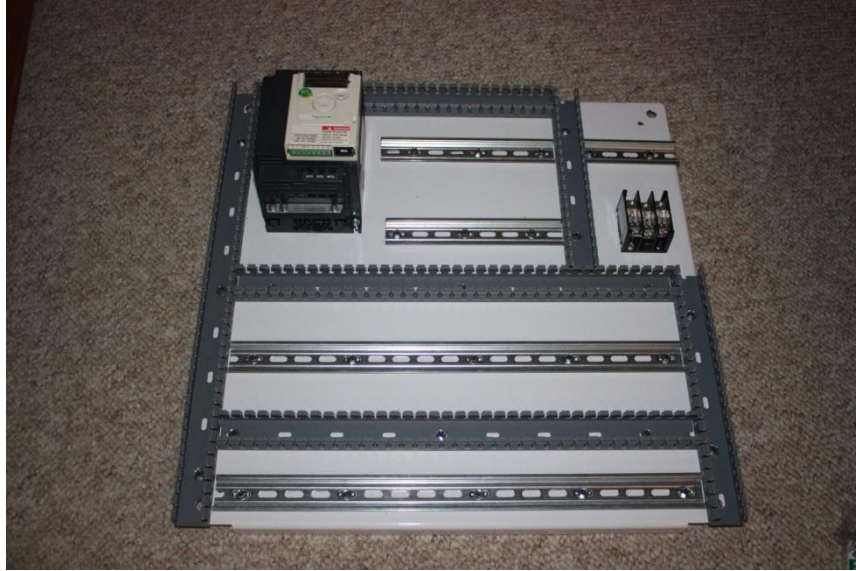
Figure 14. Subpanel with DIN rail, VFD, and distribution block mounted.
