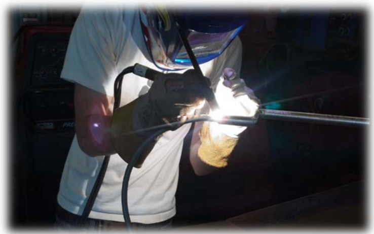
Figure 29. Simon Rowe welding the curved rail to one side of the support structure.
