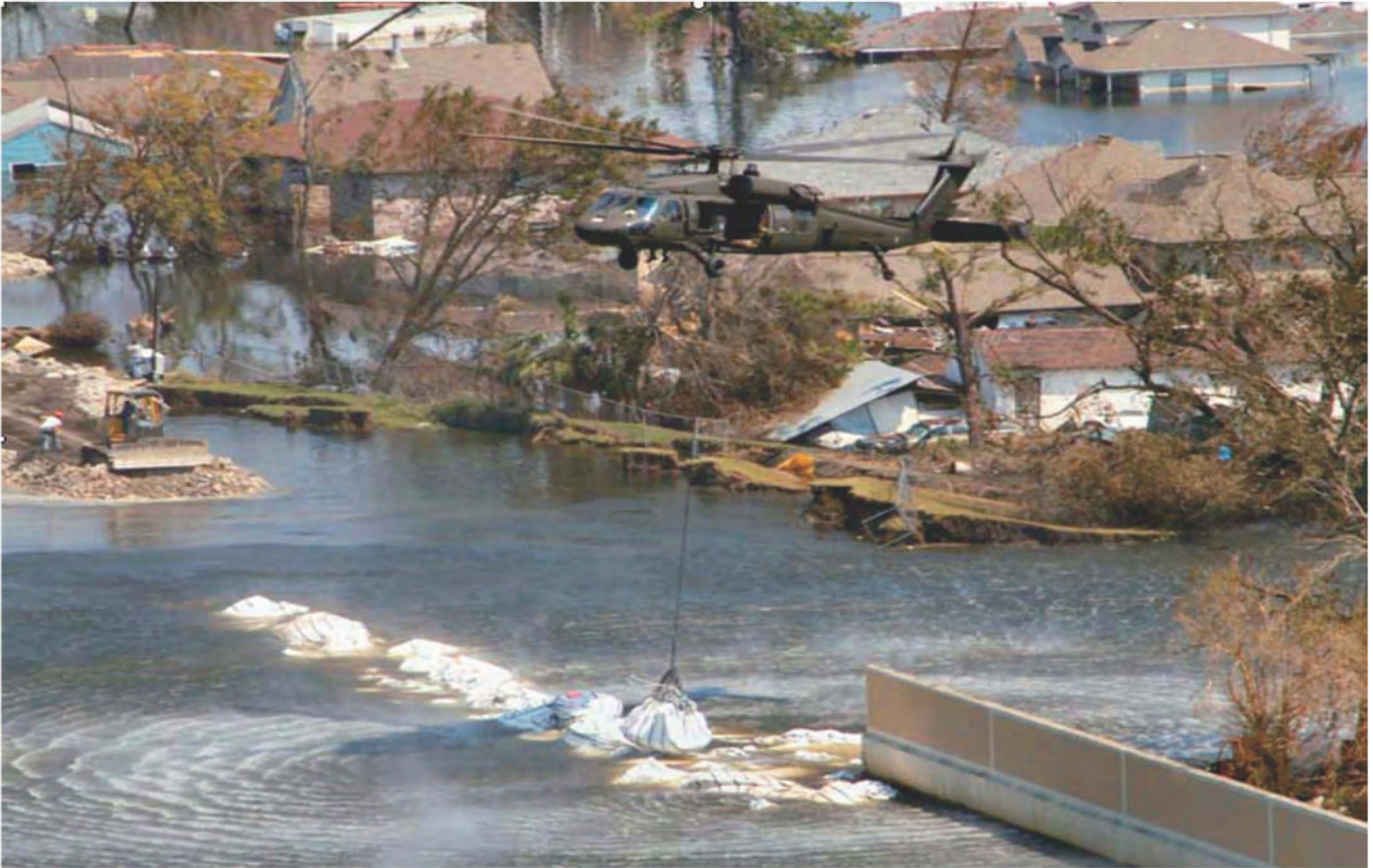
Fig. 2. (Color) Breach at the East Bank of the 17th Street Drainage Canal (USACE 1990)
