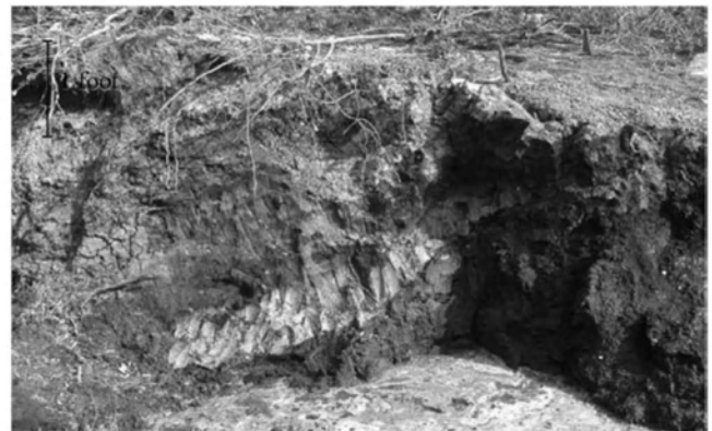
Fig. 5. View of the exit of the upper failure surface (Toe Scarp No.1), at the inboard toe of the laterally translated embankment (IPET 2006)
