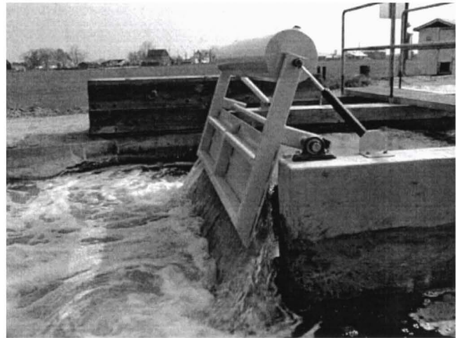
FIG. 12. Flap Gate at Turlock ID, Calif.; This Gate Was Designed without Frame, and Has a Stabilizer in Different Position Than That Shown in Fig. 1
