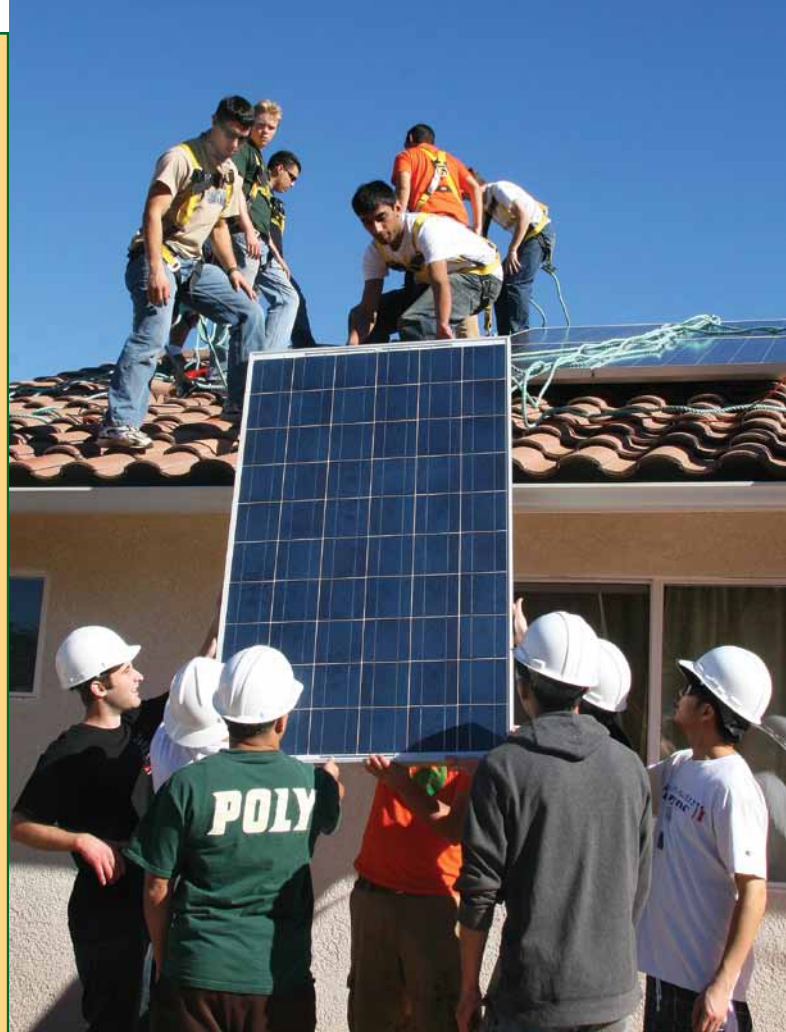
Working with the Cal Poly Power & Energy Society, engineering students lift a solar panel on the roof of a home in Nipomo.
