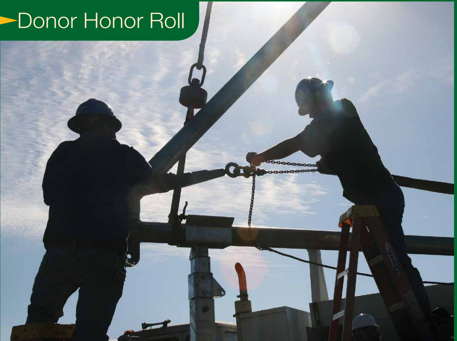
Construction workers adjust a crane used to erect the tower for the Cal Poly Wind Power project on a remote hillside on campus.
