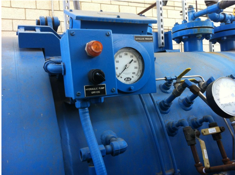
Figure 10. Hydraulic Pump Switch
